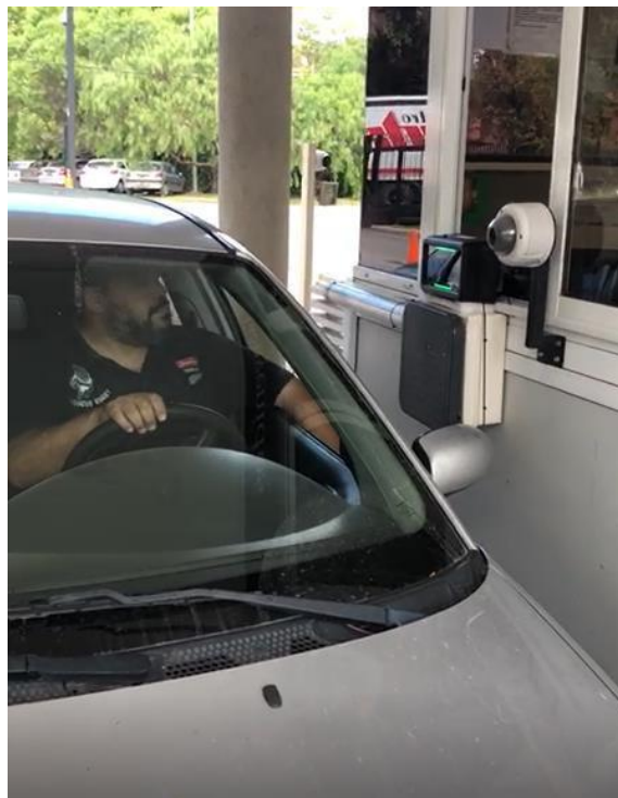
nano EXT device installed outdoors at a car port.
